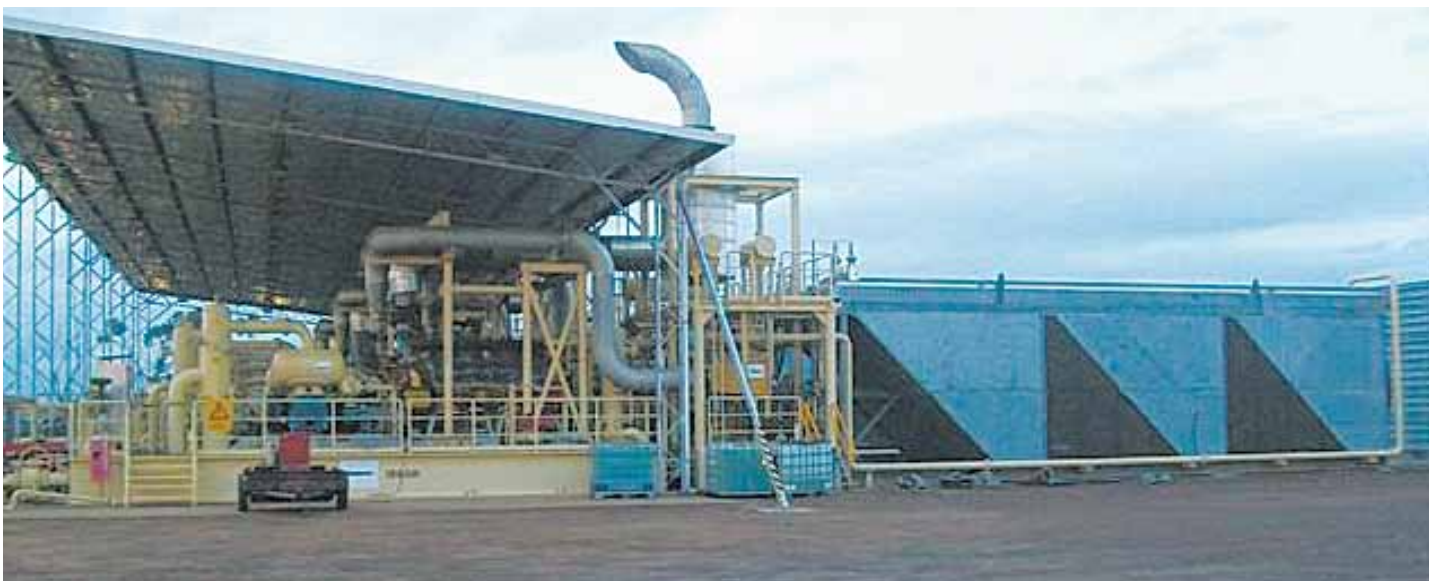
A typical Gas Compression Engine is the Caterpillar G3612. This 12 cylinder engine delivers 2647 kilowatts (equivalent to 3548 horsepower).
