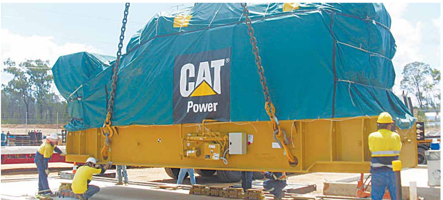
The Caterpillar G3616 Gen Set, one of only four in Australia, is unloaded on site.
