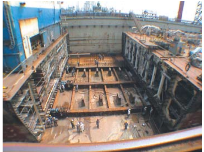
AFTER – The mid section is pre-cut to enable the upgrade and extended length.
