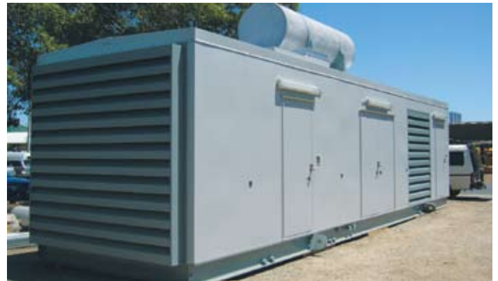
The Caterpillar 3512 Gensets are each housed in soundproof, weatherproof enclosures that can be moved to wherever power is required.
