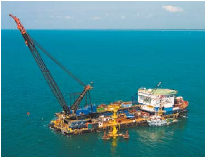
BEFORE – The 114 metre Derrick Pipe Laying Barge before the most recent upgrade.
