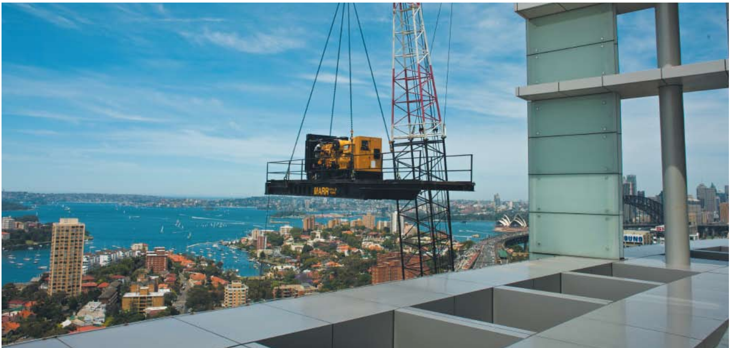
Rising to the challenge. With Caterpillar Genset delivery, installation and commissioning – in this high-rise city building – all completed the same day.
