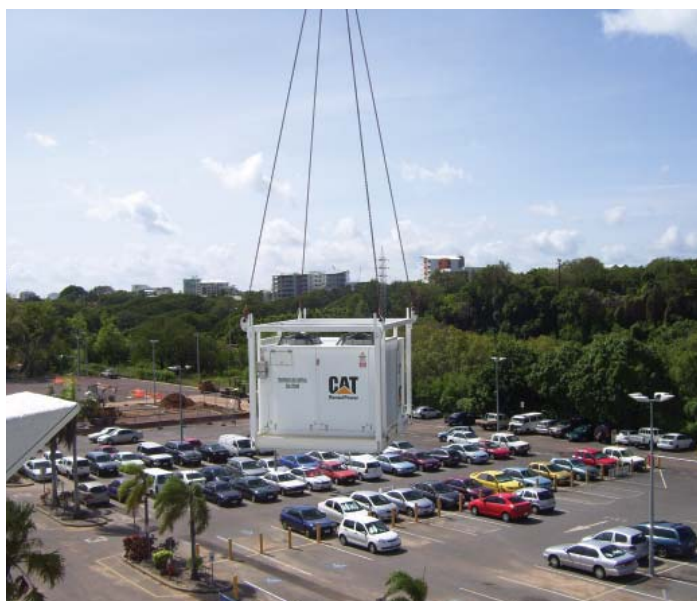
A supplementary 100KW DX air conditioning unit being lifted to the second floor of Darwin's Skycity Casino to provide cooling during the venue's refurbishment.
