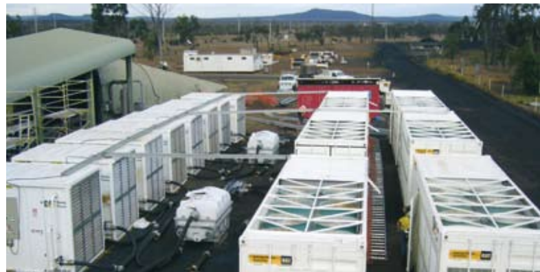
A CAT Rental Power refrigeration system is making life easier for QLD miners.
